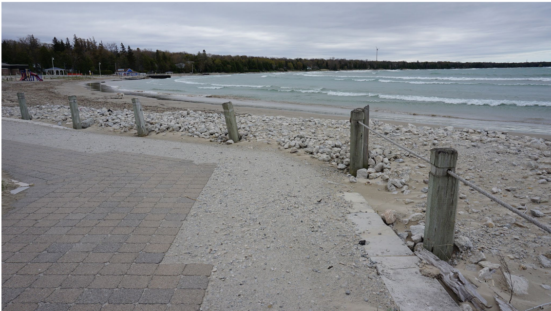
Figure 1 – Damaged Walkway, Port Elgin (April 30, 2021)
