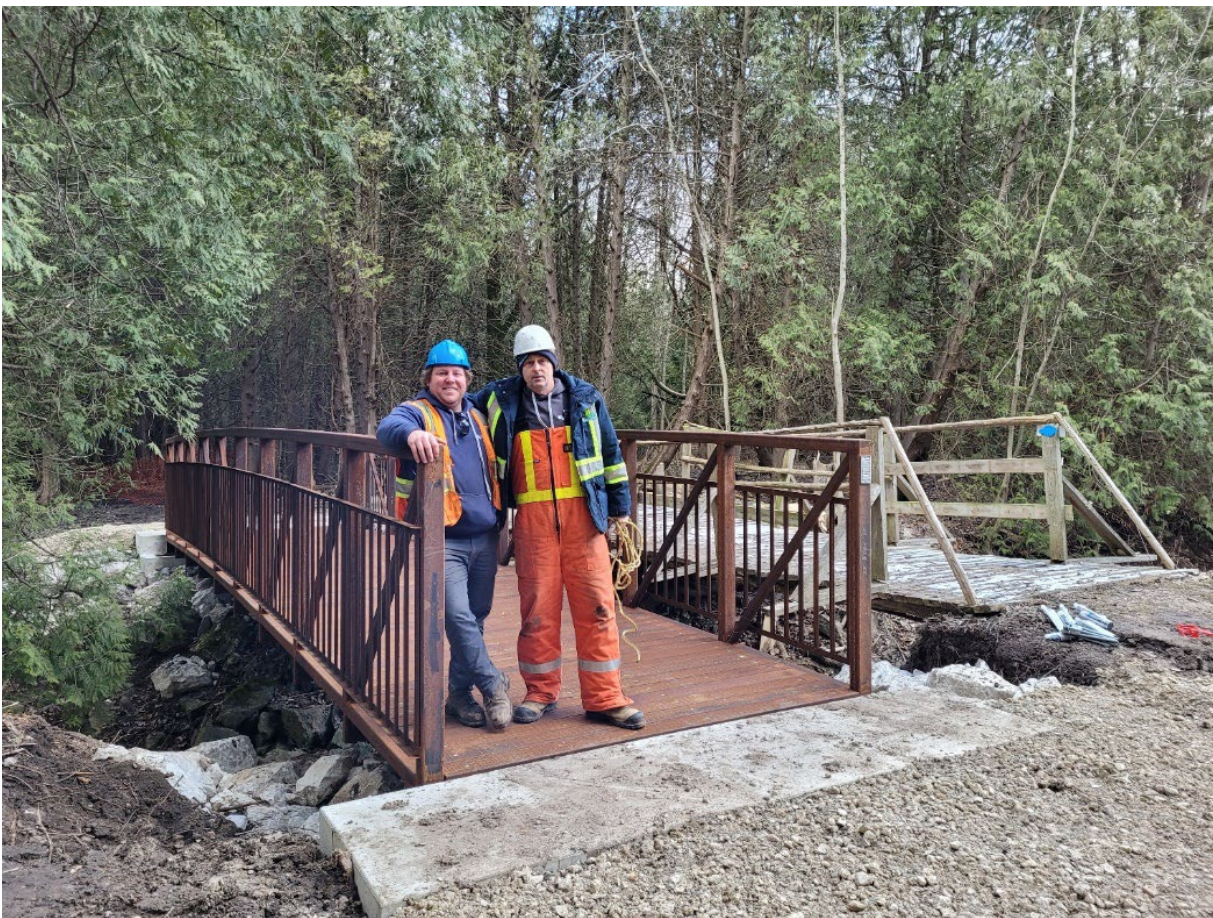
Figure 1 Anthony Quipp and Rick Rowbotham, SVCA staff, stand on newly installed iron bridge.
