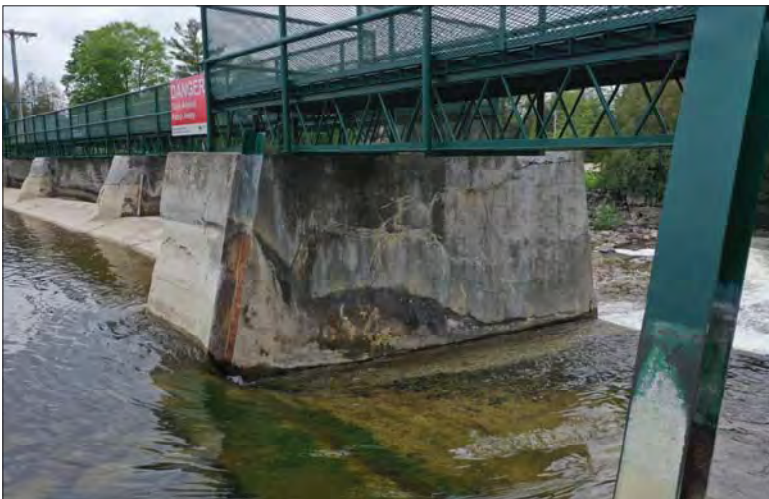
Filename: DJI_0658.JPG Photo 45 - May 15, 2024 Durham Upper Dam and Dyke Left Side of Pier 2
