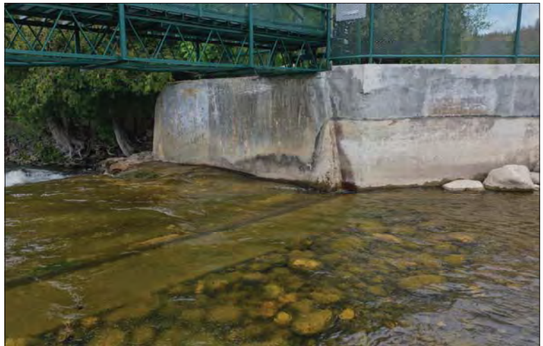
Filename: DJI_0650.JPG Photo 38 - May 15, 2024 Durham Upper Dam and Dyke Right Side of Left Abutment
