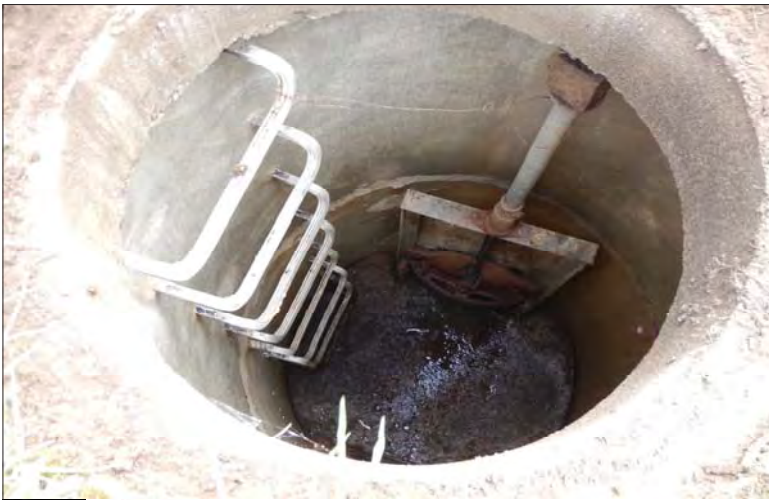
Filename: DSCN8056.JPG Photo 103 - May 15, 2024 Durham Upper Dam and Dyke Manhole Structure in Dyke
