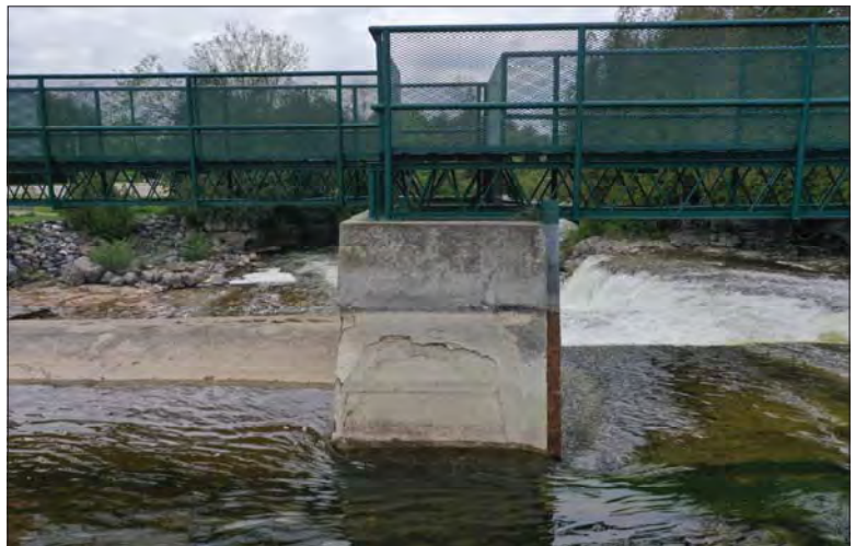
Filename: DJI_0659.JPG Photo 46 - May 15, 2024 Durham Upper Dam and Dyke Upstream Side of Pier 2
