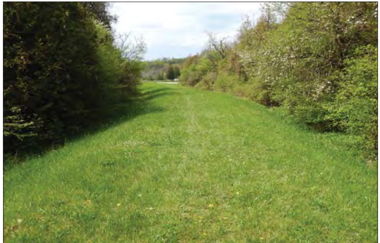
Filename: DSCN8073.JPG Photo 112 - May 15, 2024 Durham Upper Dam and Dyke Crest of Dyke Looking Towards Dam
