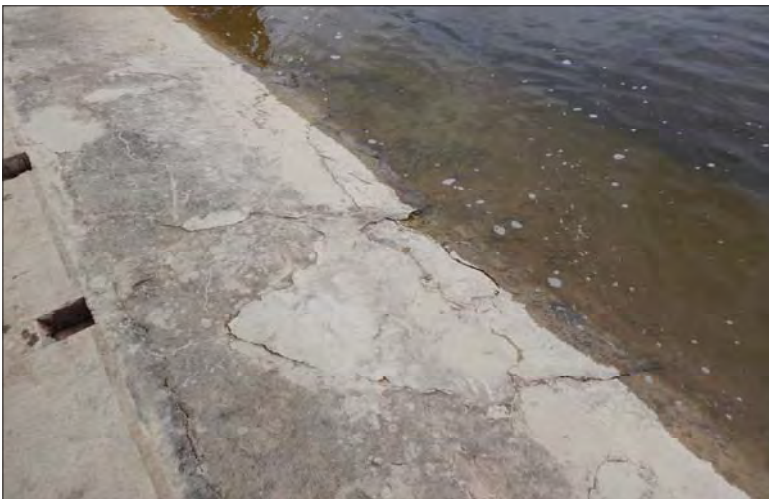
Filename: DSCN7969.JPG Photo 51 - May 15, 2024 Durham Upper Dam and Dyke Delamination and Spalling on Upstream Apron, Sluiceway 3
