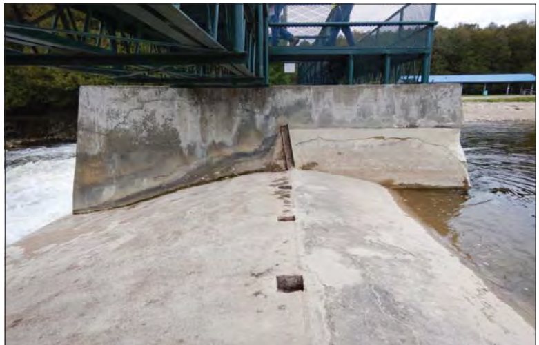
Filename: DSCN7972.JPG Photo 48 - May 15, 2024 Durham Upper Dam and Dyke Right Side of Pier 2
