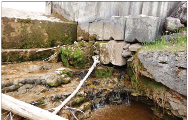
Filename: DSCN7929.JPG Photo 4 - May 15, 2024 Durham Upper Dam and Dyke Seepage on Right Side of Dam
