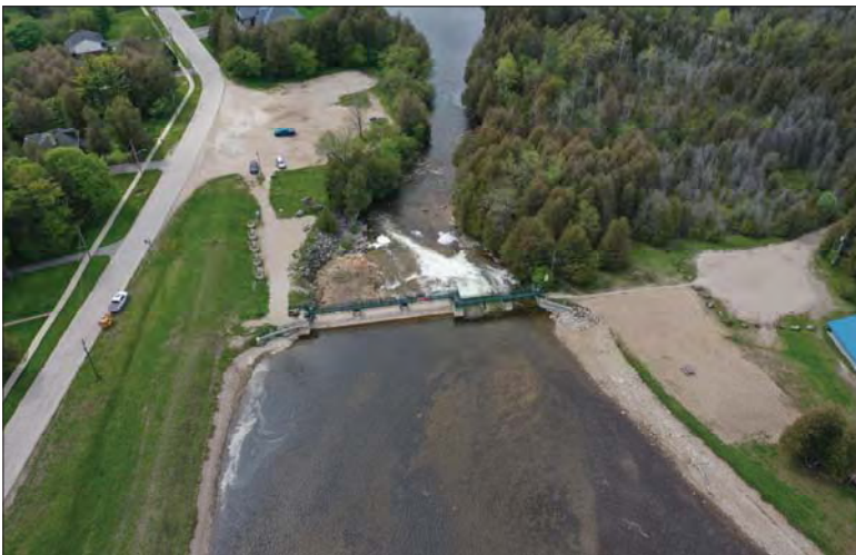
Filename: DJI_0691.JPG Photo 33 - May 15, 2024 Durham Upper Dam and Dyke Aerial View of Upstream Side of Dam
