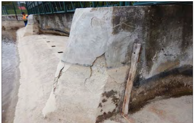
Filename: DSCN7967.JPG Photo 54 - May 15, 2024 Durham Upper Dam and Dyke Delamination and Spalling on Upstream Side of Pier 3
