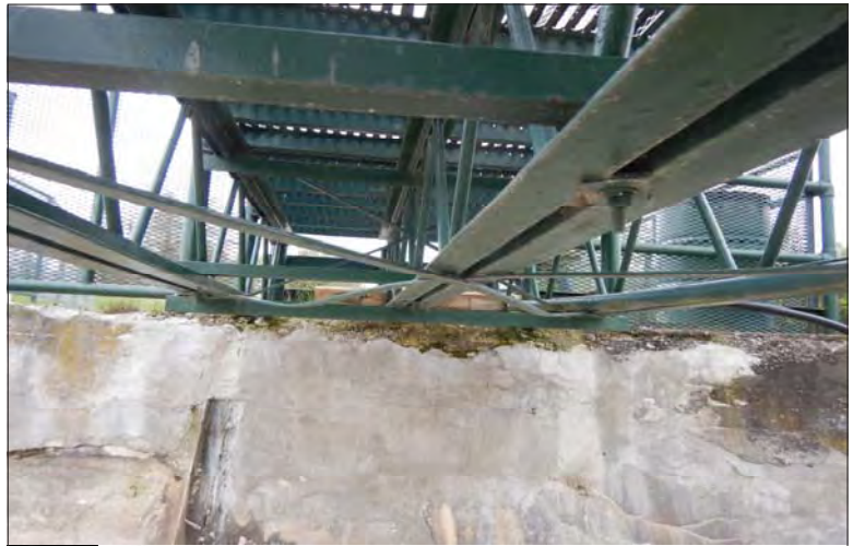
Filename: DSCN7945.JPG Photo 84 - May 15, 2024 Durham Upper Dam and Dyke Underside of Pedestrian Walkway
