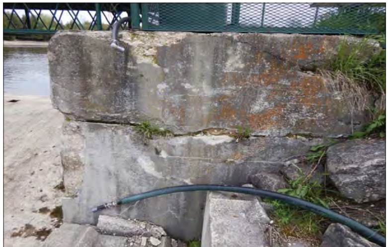
Filename: DSCN7985.JPG Photo 6 - May 15, 2024 Durham Upper Dam and Dyke Downstream Side of Right Abutment
