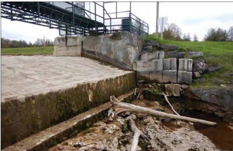
Filename: DSCN7936.JPG Photo 3 - May 15, 2024 Durham Upper Dam and Dyke Left Side of Right Abutment
