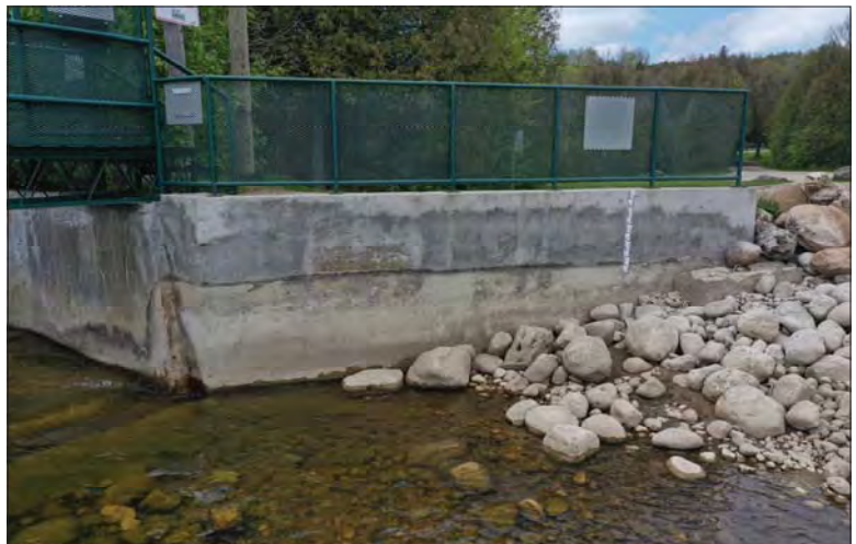
Filename: DJI_0649.JPG Photo 36 - May 15, 2024 Durham Upper Dam and Dyke Upstream Left Wingwall
