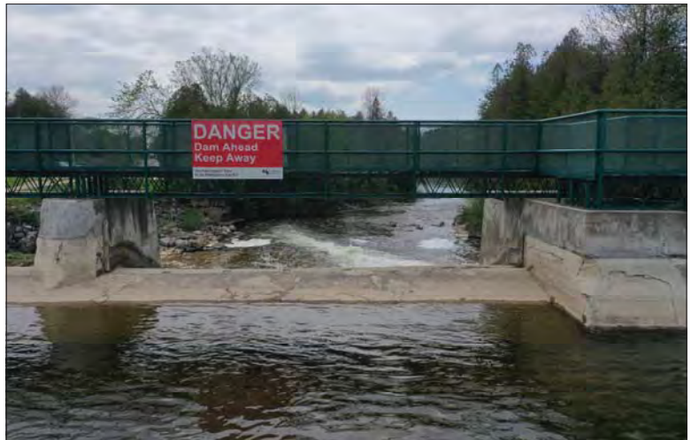
Filename: DJI_0678.JPG Photo 50 - May 15, 2024 Durham Upper Dam and Dyke Upstream Side of Sluiceway 3
