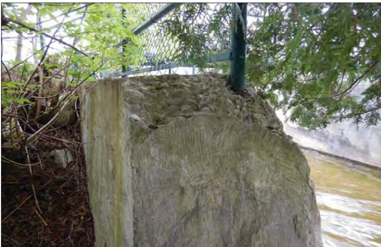
Filename: DSCN8099.JPG Photo 27 - May 15, 2024 Durham Upper Dam and Dyke Spill on Downstream Side of Left Abutment
