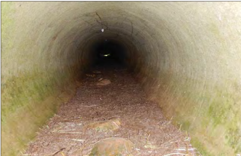
Filename: DSCN8061.JPG Photo 105 - May 15, 2024 Durham Upper Dam and Dyke Inside Outlet Pipe
