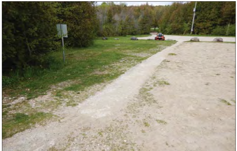
Filename: DSCN8023.JPG Photo 92 - May 15, 2024 Durham Upper Dam and Dyke Left Embankment and Overflow Spillway
