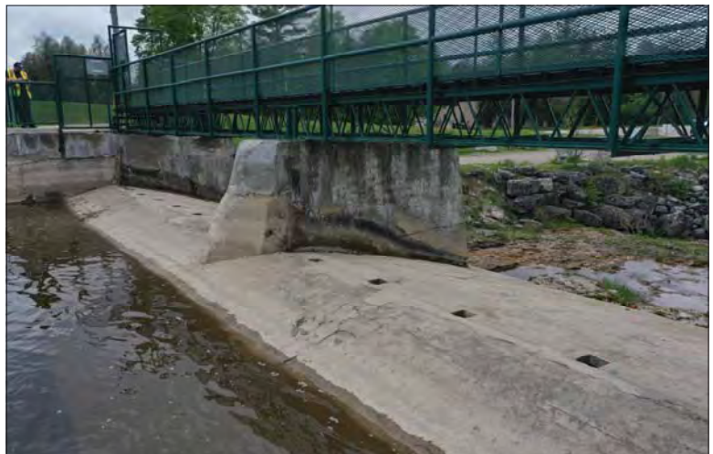
Filename: DJI_0665.JPG Photo 60 - May 15, 2024 Durham Upper Dam and Dyke Left Side of Pier 4
