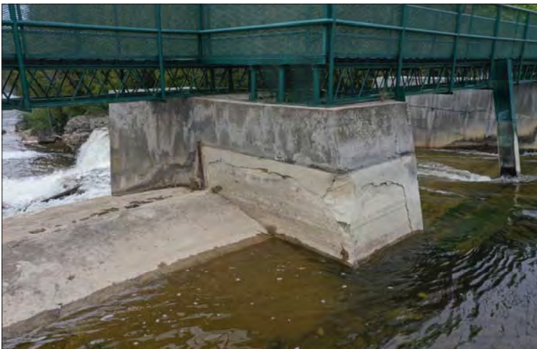
Filename: DJI_0660.JPG Photo 47 - May 15, 2024 Durham Upper Dam and Dyke Right Side of Pier 2
