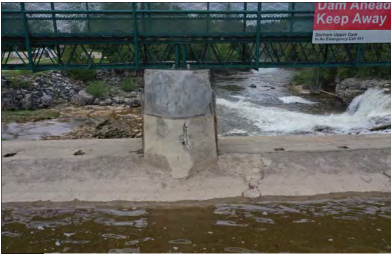
Filename: DJI_0663.JPG Photo 55 - May 15, 2024 Durham Upper Dam and Dyke Upstream Side of Pier 3
