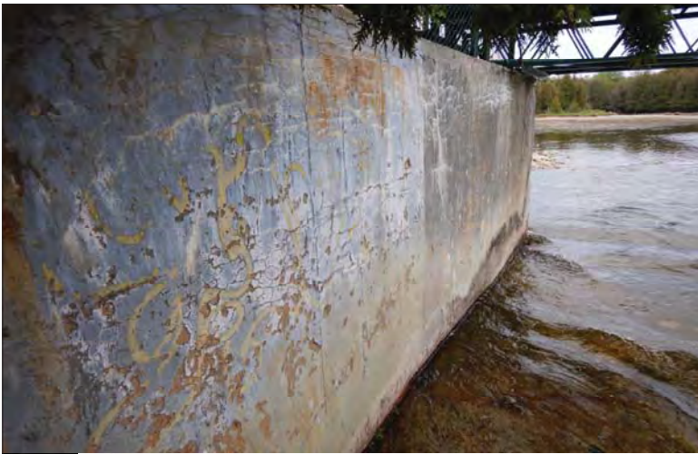
Filename: DSCN8101.JPG Photo 25 - May 15, 2024 Durham Upper Dam and Dyke Right Side of Left Abutment
