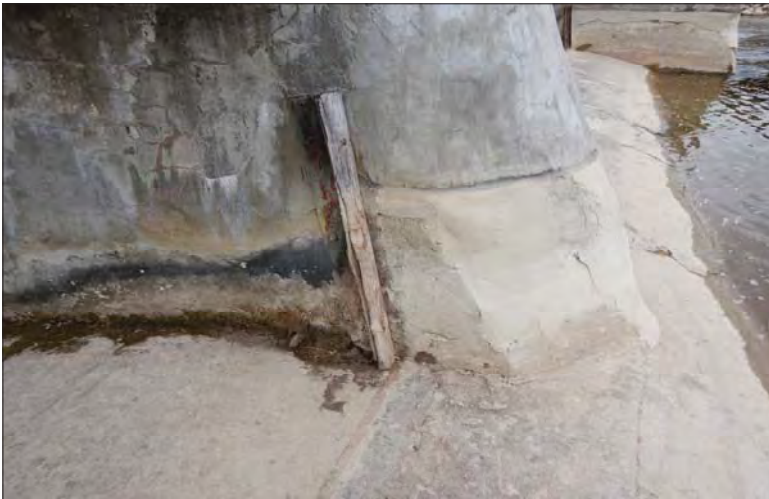
Filename: DSCN7963.JPG Photo 57 - May 15, 2024 Durham Upper Dam and Dyke Stoplog Gain in Right Side of Pier 3
