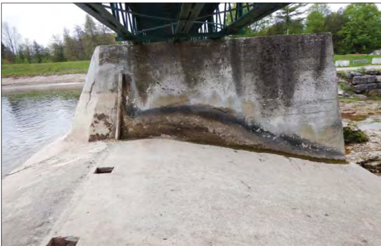
Filename: DSCN7971.JPG Photo 53 - May 15, 2024 Durham Upper Dam and Dyke Left Side of Pier 3
