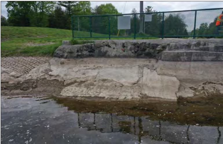
Filename: DJI_0671.JPG Photo 69 - May 15, 2024 Durham Upper Dam and Dyke Upstream Right Wingwall
