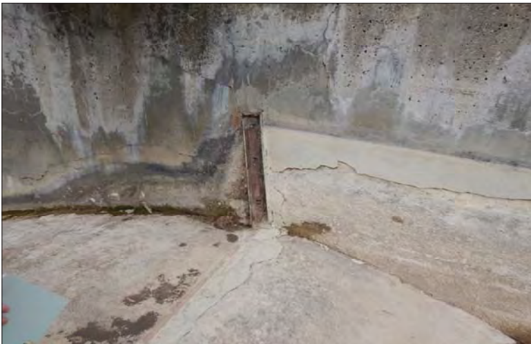
Filename: DSCN7982.JPG Photo 49 - May 15, 2024 Durham Upper Dam and Dyke Stoplog Gain in Right Side of Pier 2
