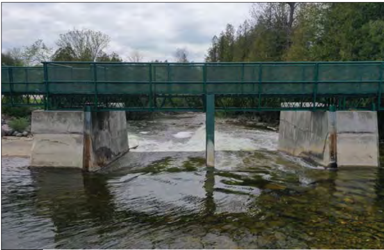
Filename: DJI_0679.JPG Photo 43 - May 15, 2024 Durham Upper Dam and Dyke Upstream Side of Sluiceway 2
