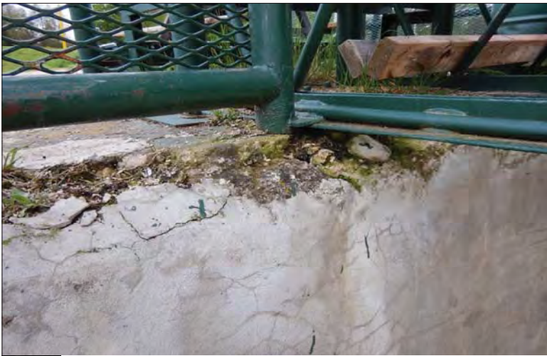
Filename: DSCN7947.JPG Photo 85 - May 15, 2024 Durham Upper Dam and Dyke Walkway Anchor in Right Abutment
