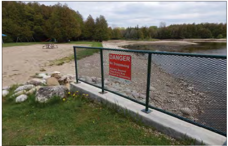
Filename: DSCN8021.JPG Photo 90 - May 15, 2024 Durham Upper Dam and Dyke Railing on Upstream Left Wingwall
