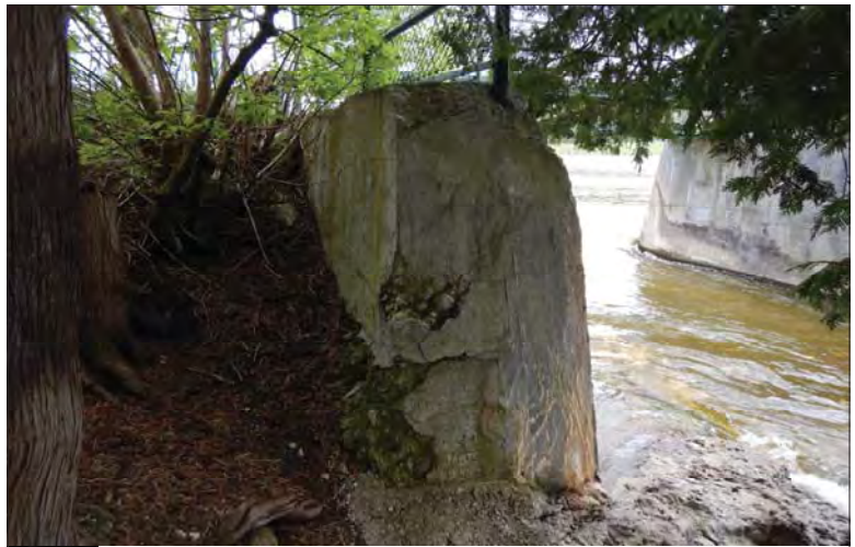
Filename: DSCN8097.JPG Photo 26 - May 15, 2024 Durham Upper Dam and Dyke Downstream Side of Left Abutment
