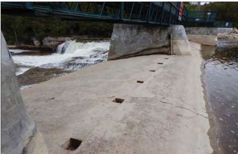
Filename: DSCN7958.JPG Photo 59 - May 15, 2024 Durham Upper Dam and Dyke Upstream Apron, Sluiceway 4
