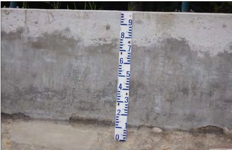
Filename: DSCN8029.JPG Photo 37 - May 15, 2024 Durham Upper Dam and Dyke Staff Gauge on Upstream Left Wingwall
