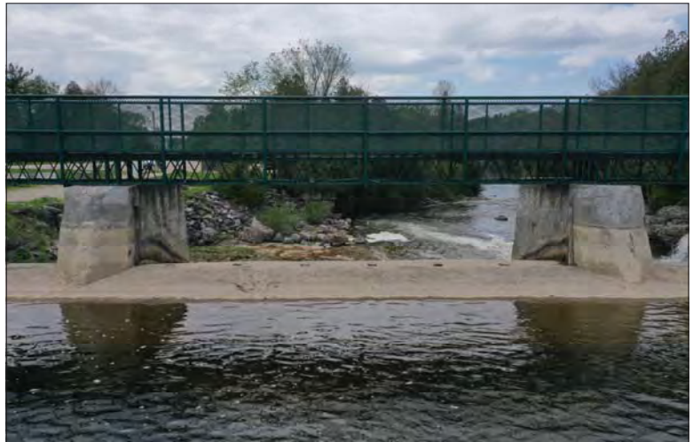
Filename: DJI_0677.JPG Photo 58 - May 15, 2024 Durham Upper Dam and Dyke Upstream Side of Sluiceway 4
