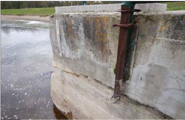
Filename: DSCN7948.JPG Photo 67 - May 15, 2024 Durham Upper Dam and Dyke Railing Anchor on Right Abutment
