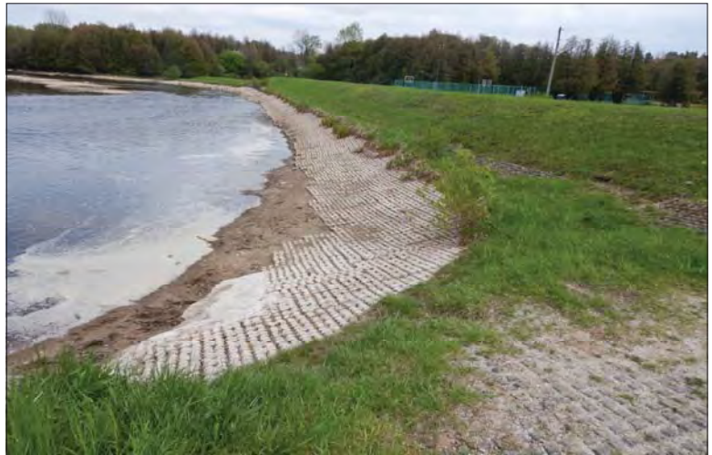
Filename: DSCN8037.JPG Photo 70 - May 15, 2024 Durham Upper Dam and Dyke Erosion Protection on Left Side of Dyke
